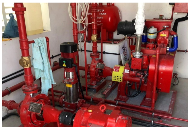
FIRE PUMP ROOM — COMMISSIONED
